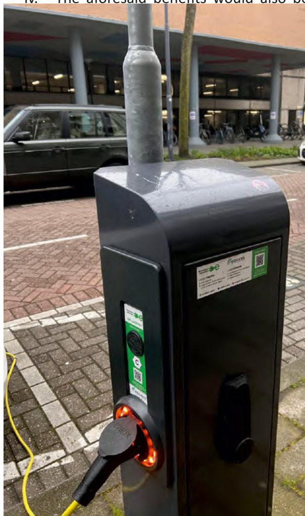
EV Charging Station
