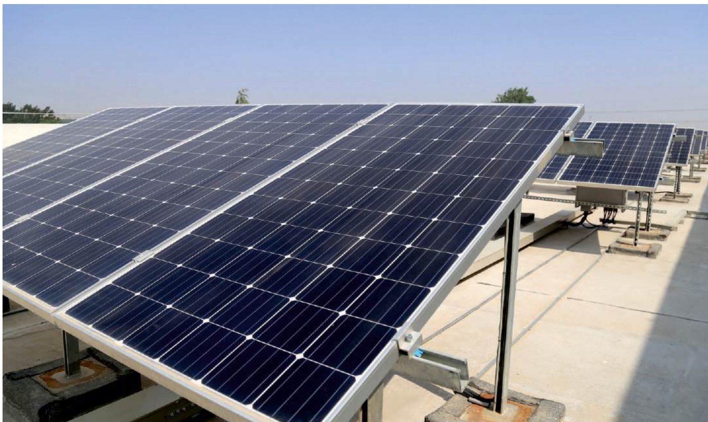
Solar Rooftop Plant
