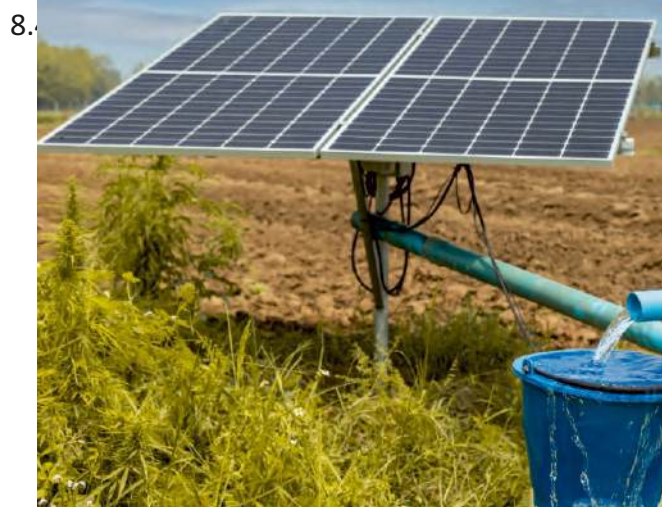
Off Grid Stand Alone Solar Pump
