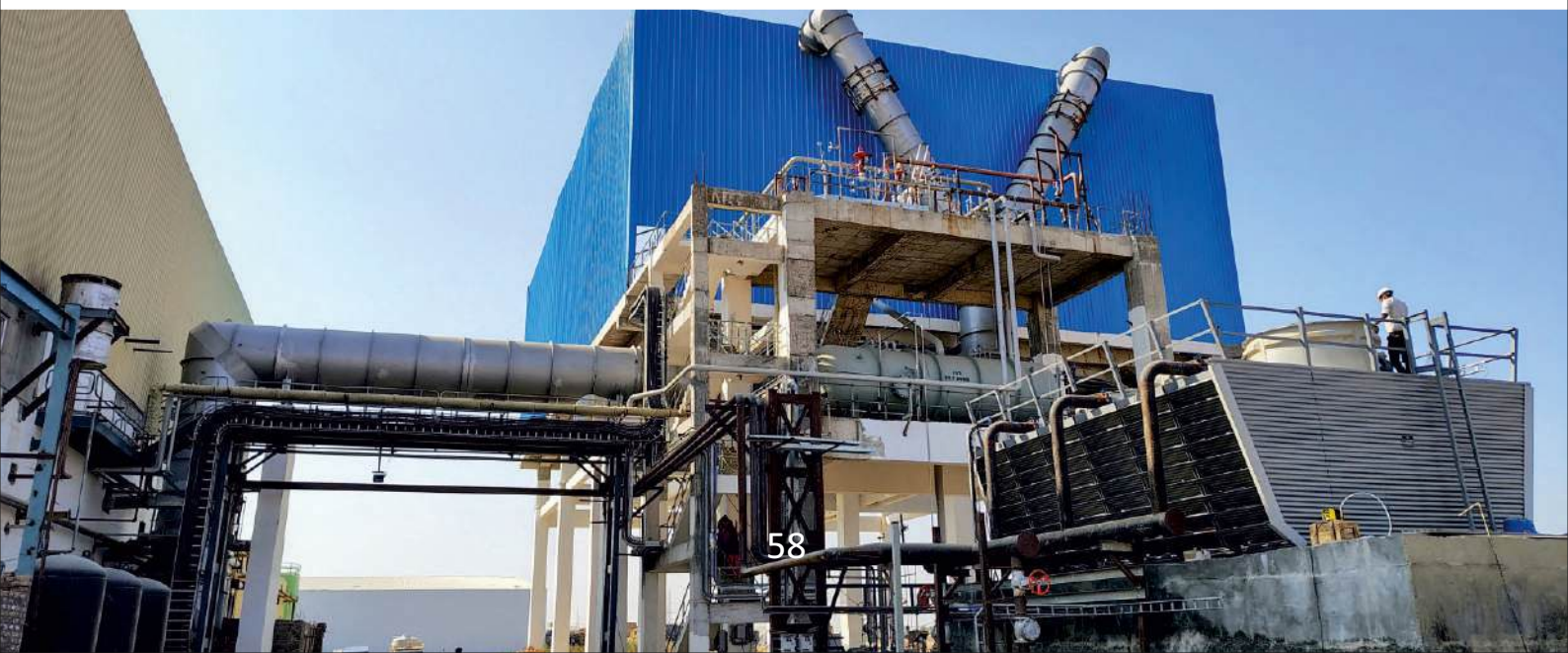
Biomass Plant - Chattargarh, Bikaner
